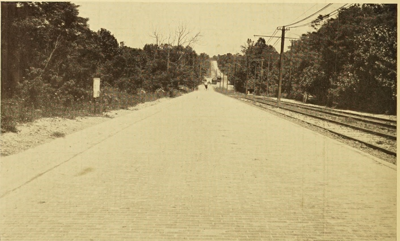
CONDITION OF BRICK SURFACE IN JUNE, 1913
